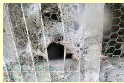
Damage to poultry house wire mesh.
