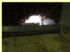
Holes in poultry house walls
